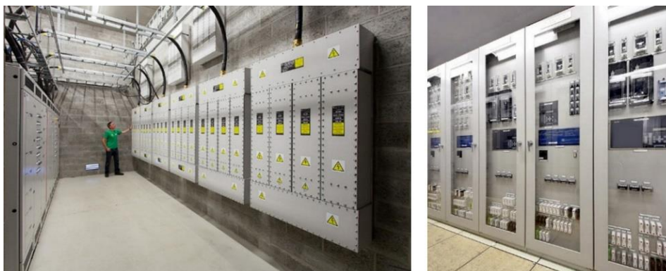
Figure1. HEMP filters (left) and control cabinets (right). For size comparison.
