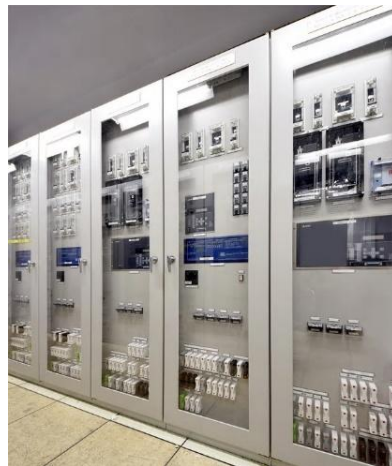
Figure1. Electronic equipment controls cabinets used in the power industry
