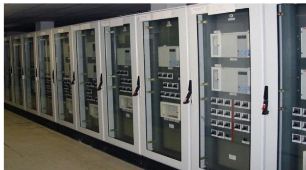
Figure1. Common placement of electronic equipment, in particular, digital protection relay (DPR) in glass-door cabinets.
