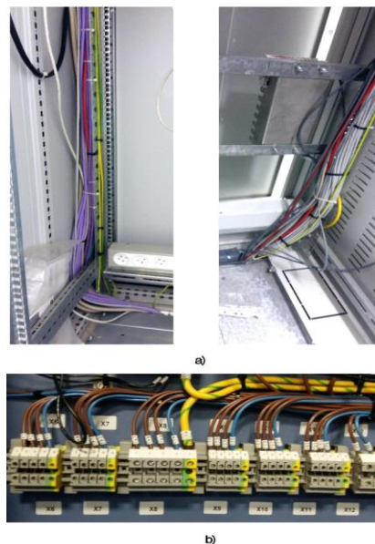
Figure10. There are two main principles of cable entry into a cabinet: a) external cables are laid through the whole cabinet and then they are connected directly to electronic equipment's terminals; b) external cables are connected through intermediate terminals at the cabinet's entrance.
