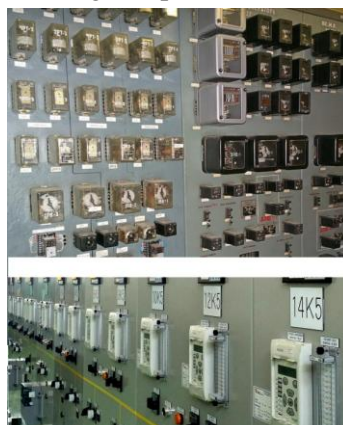
Figure1. Relay protection panels: electromechanical (above) and microprocessor-based (below).
