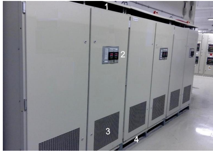
Fig1. Design of power plant's BC. The figures indicate the “weaknesses” of cabinets that allow unobstructed access of HEMP inside the cabinet.
