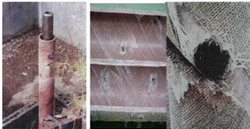
Figure8. Results of Perforation of Fiberglass Casing
