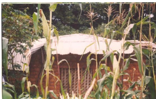
Plate2. Abandoned Palace of Bongala Note the dilapidated roof and the maize plants
