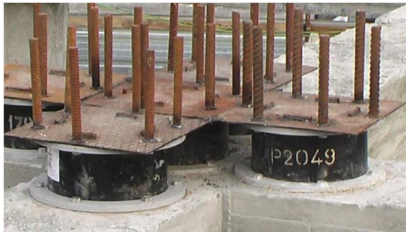
Figure8. View of the upper sockets with anchor rods installed above the seismic isolators
