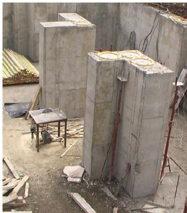
Figure6. Columns with the L-shaped cross section constructed in the basement with two or three seismic isolators' lower sockets on top of them
