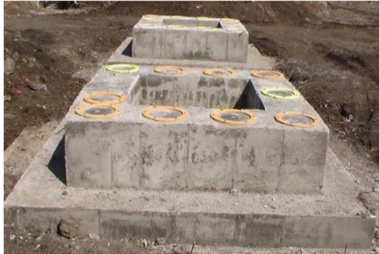
Figure7. View of the constructed foundation under the hollow columns to support the so called “bridge”. Ten seismic isolators’ lower sockets are placed on each foundation of the four hollow columns
