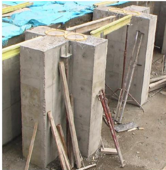
Figure5. Columns with the T-shaped cross section constructed in the basement with two seismic isolators' lower sockets on top of them
