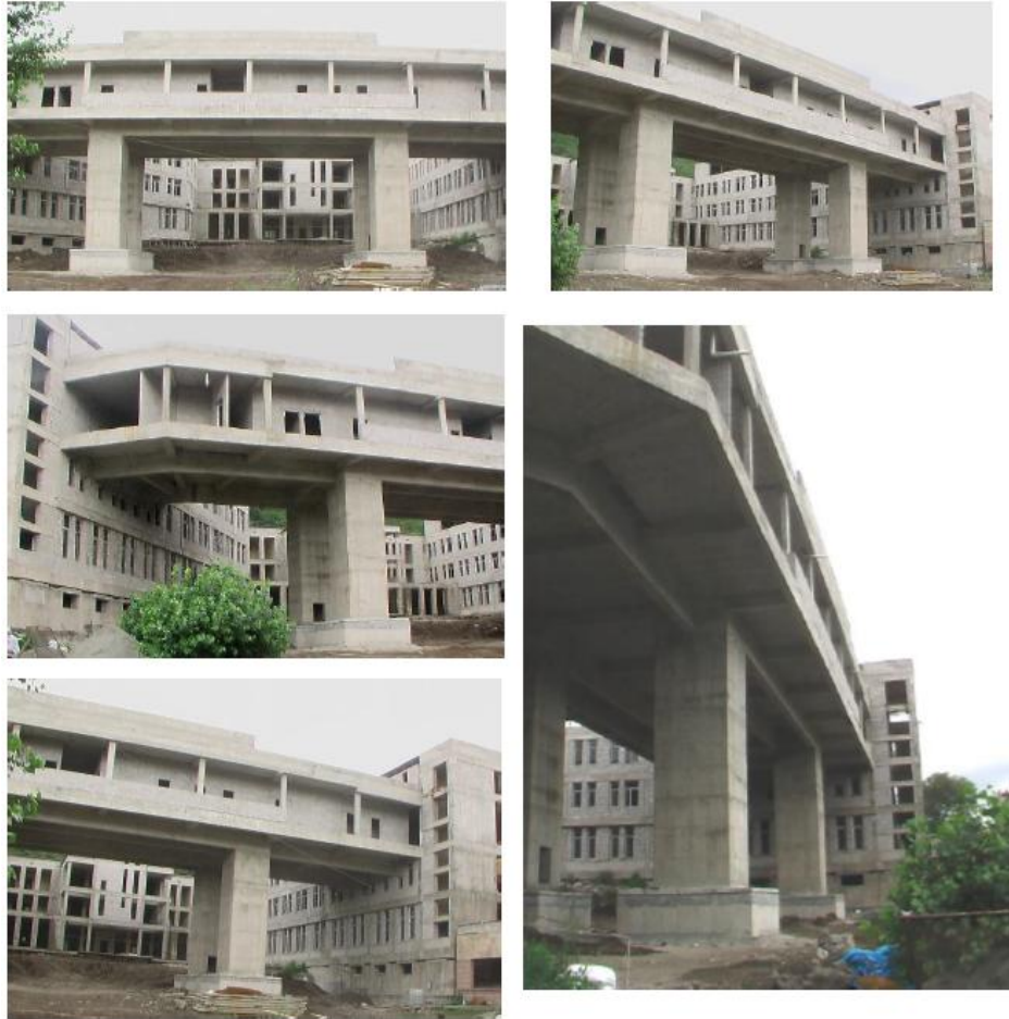
Figure11. The views of the four hollow columns supporting the fourth floor (“bridge”) of the superstructure connecting the left and right wings of base isolated hospital building
