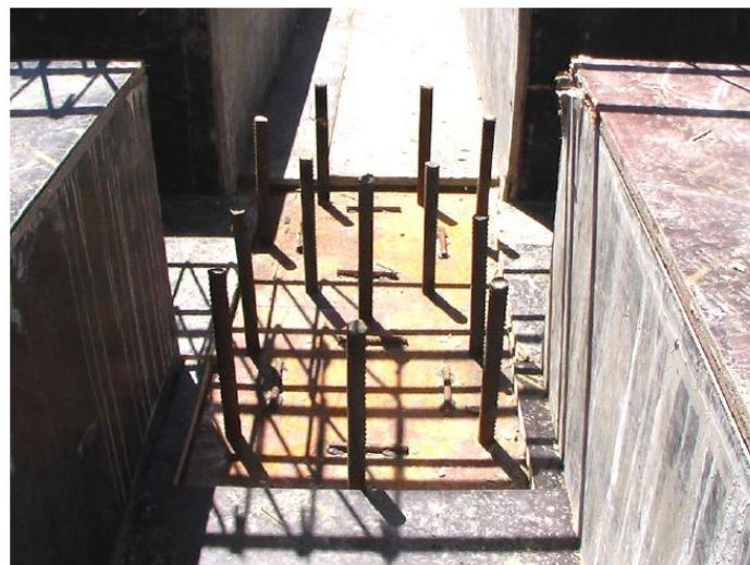
Figure9. View of the wooden forms of upper beams to be constructed immediately above the seismic isolators. Anchor rods of upper sockets will be anchored in the upper beams
