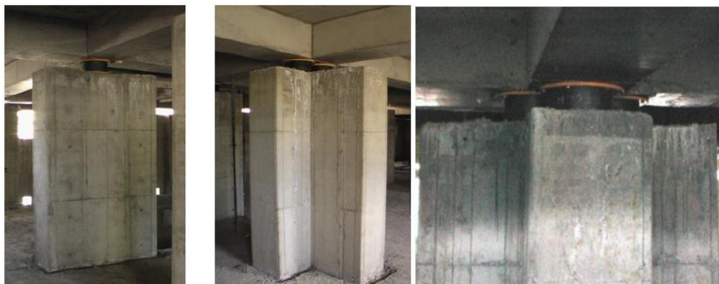
Figure3. Examples on installation of rubber bearings’ clusters in the 4 - story base isolated hospital building “Vanadzor” during construction
