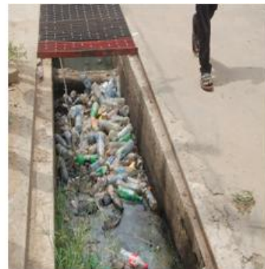
Figure2. Blocked Drainage by debris
