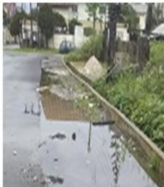
Fig1. Kerb higher than the pavement without inlets
