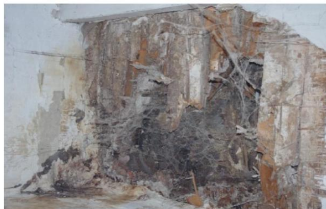
Figure4. Damage due to roof leakage
